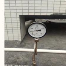
改善後熱水供水壓力0.2Mpa
